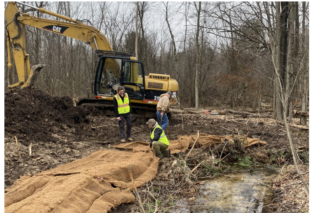
Subcontractor Kanouse Outdoor Restoration and design engineering firm GEI implementing habitat restoration down stream of Pierce Rd on Swinton Creek.
