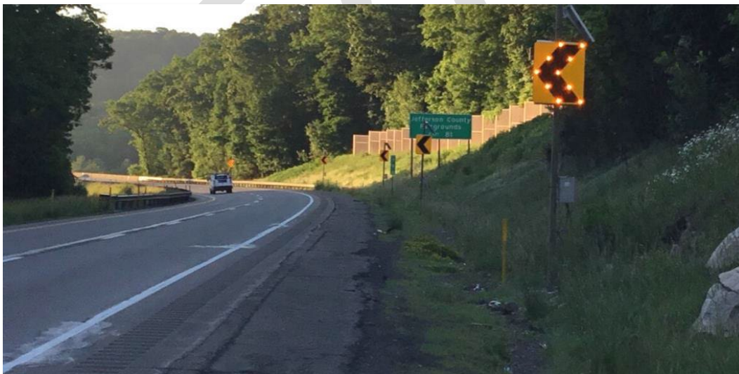
Figure 27 - LED Chevron Sign (PennDOT)
