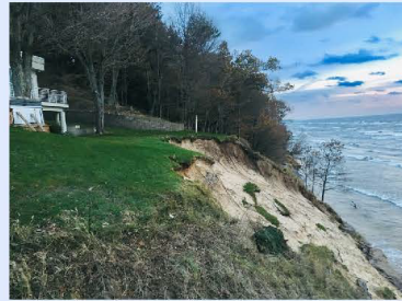
Erosion at a residence on the Lake Michigan Shoreline in the City of Norton Shores, Muskegon County.
