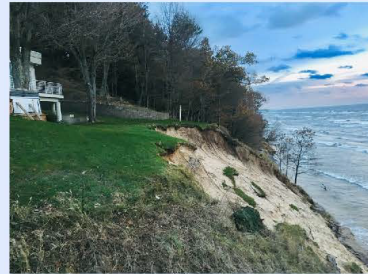
Erosion at a residence on the Lake Michigan Shoreline in the City of Norton Shores, Muskegon County.
