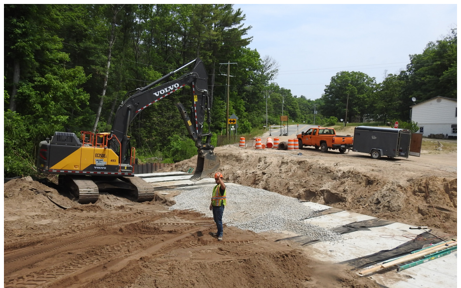
Construction activities at Sweeter Road and Little Cedar Creek crossing on June 6, 2023.
