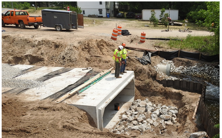
Additional construction activities, at Sweeter Road and Little Cedar Creek crossing on June 6, 2023.
